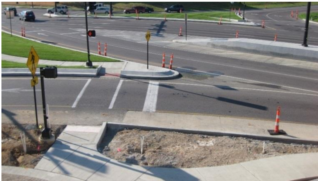
Exhibit 7-15 Pedestrian Signal and Push Button for Left- Turn onto Freeway (Pedestrian Facility on Outside)
