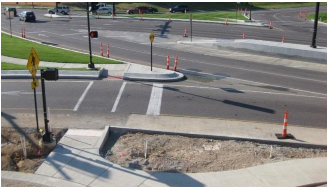
Exhibit 7-15 Pedestrian Signal and Push Button for Left- Turn onto Freeway (Pedestrian Facility on Outside)
